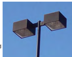
Shoe-box lighting or other downcast fixtures to be used in large parking areas
